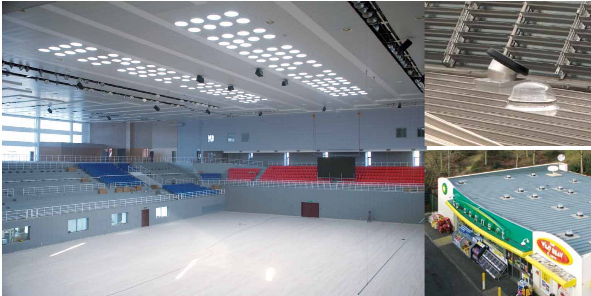
ABOVE: 148 Solatube® 330 DS Daylighting Systems installed in the Judo/Taekwondo arena for the Beijing Olympics
